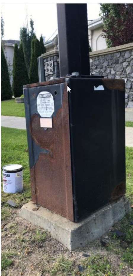
Electrical boxes before...
